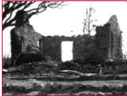
A little preventative maintenance can save you from having to come home to this. Above photo shows a home in the Crest area recently destroyed by Wildfire.
